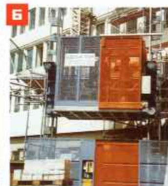
6 When the cage moves into the ground station, the cage door at the front is unlocked automatically and can be opened together with the sliding door of the ground station.
